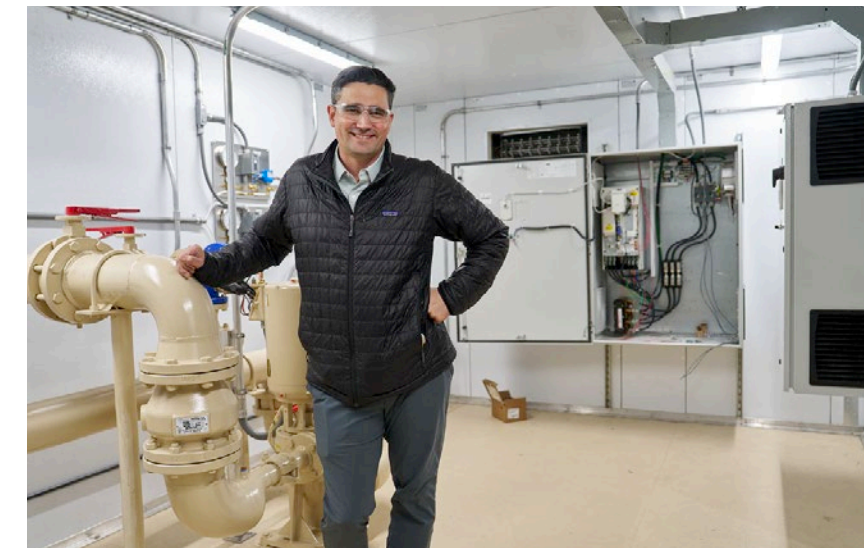
Sean Rezin is making a real success of Usemco. The company manufactures prefabricated, enclosed pump stations for municipal water management.
